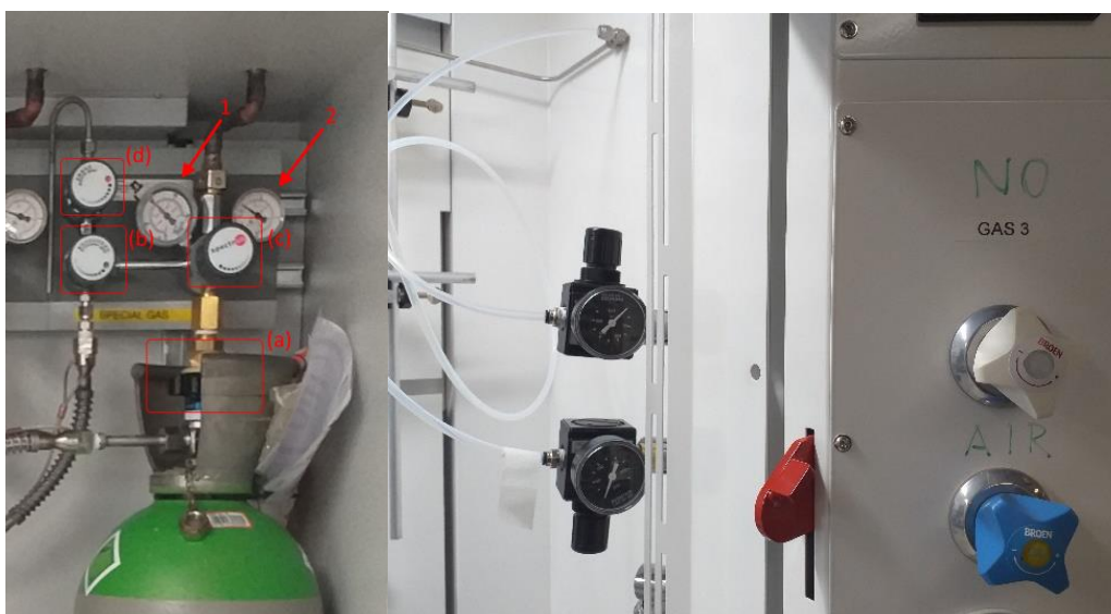
Figure 3. The regulator inside the gas cylinder cabinet (left), and the regulators and knobs in the fume hood (right)
