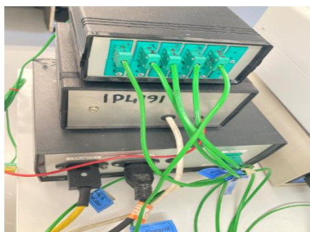
Back side of bubbler temperature display and CVD reactor temperature control box.
