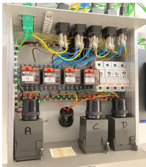
Insides of electric connections of heating line temperature control box and bubbler temperature control box
