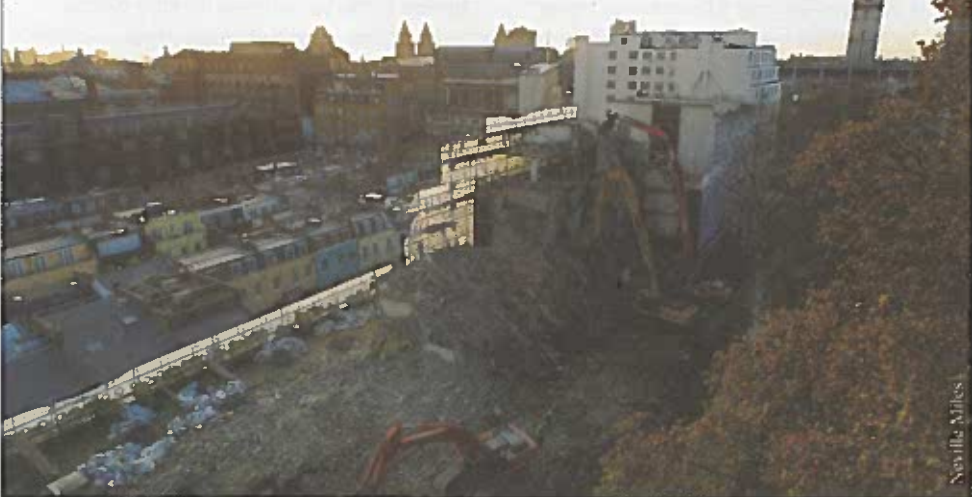
Last month saw the last of Southside demolished and the rubble removed from the site. See page three for the winners of the time capsule competition.
