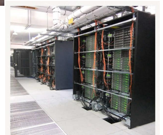
HPC Computer Room
