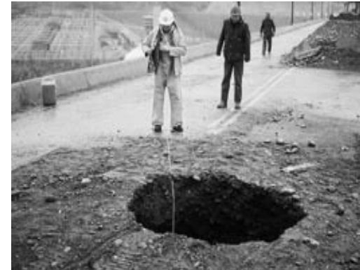
1996 Sinkhole at WAC Bennett Dam (BC Hydro as cited by Muir Wood, 2007)
